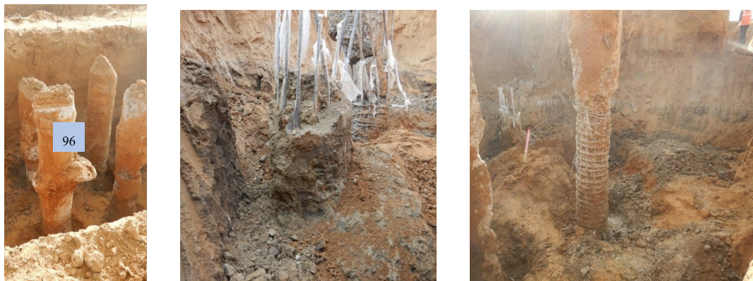
Pile 96 Pile 108 Pile 113 Bulging at shallow depth in Pile 96 Poor concrete quality in Pile 108 Exposed reinforcement in Pile 113
